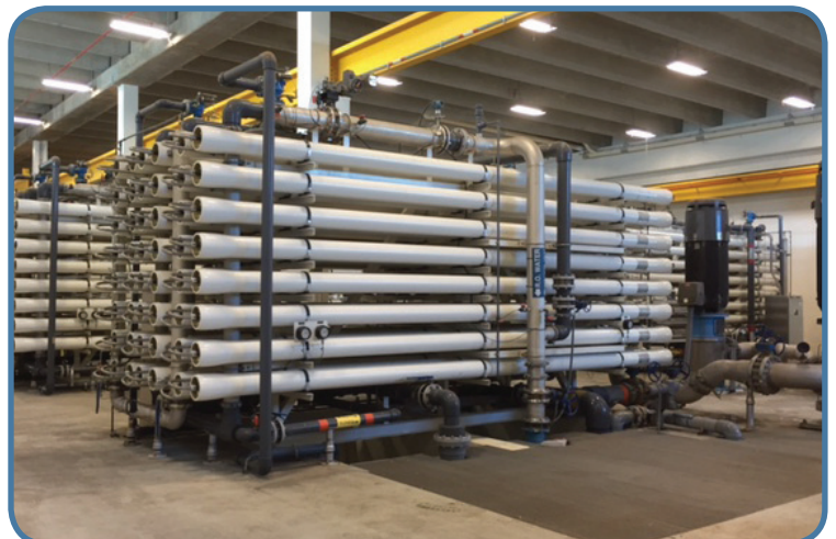
RO Trains for Reverse Osmosis
