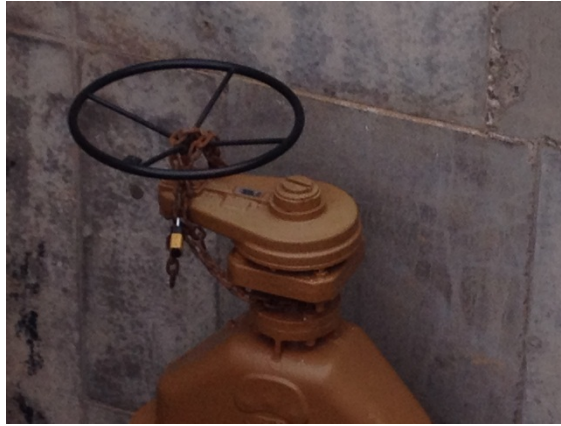
Photograph of chained valve from Headquarters PS
